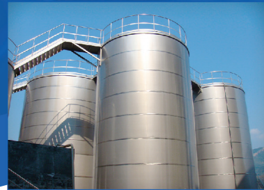
Bacs (Storage tanks)
